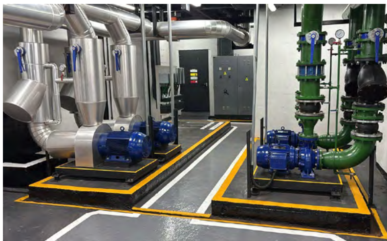
Chilled-water plant at Iguatemi Esplanada
