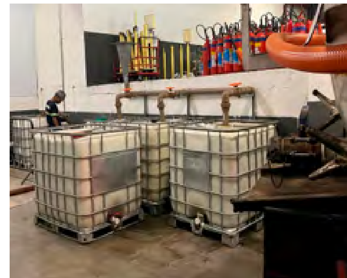
Storage pumps for wax-waste treatment
